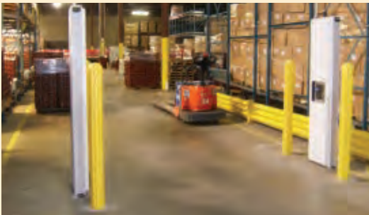
RFID technology is used to track nearly 20,000 returnable containers a day at Mission Foods.
